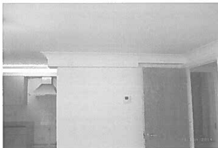
Figure 2 - A Typical Flat at Parkside Tower Post Sprinkler Installation
