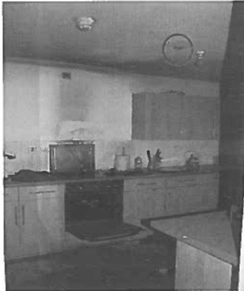
Photograph 2 - Supressed Chip Pan Fire in a Flat (sprinkler head circled)
